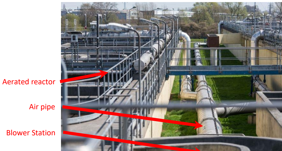
Fig. 31. Picture of reactors in Płaszów WWTP with air pipes in the first plan 5
